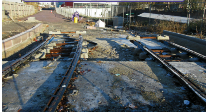
Track laying at the Dudley Castle station site in Station Drive in December 2022
